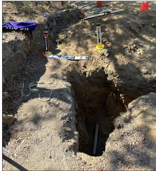
[Location of damaged wire]
